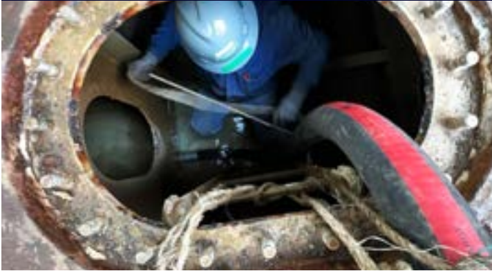
Pumping Fuel Tank
