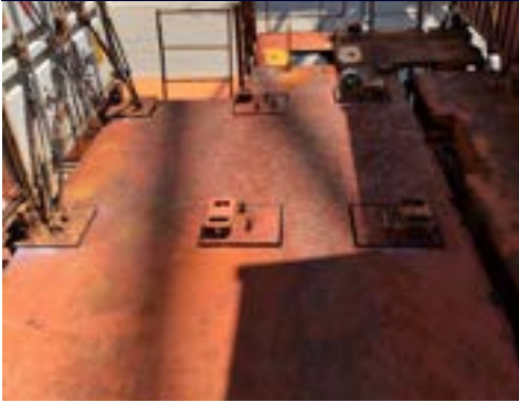
Damaged Lashing Platform
